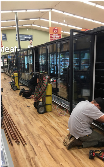
Key Mechanical teams work quickly to install a row of cases before the Goose opens for the day.
