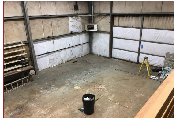
The property at 5781 Bayview Road required extensive cleaning and repairs before Whidbey Island Kayaking could join the Bayview family.
