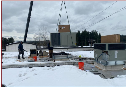
The team of Five Star Mechanical lifting new HVAC equipment onto the roof of the Cash Store during snow and power outages.
