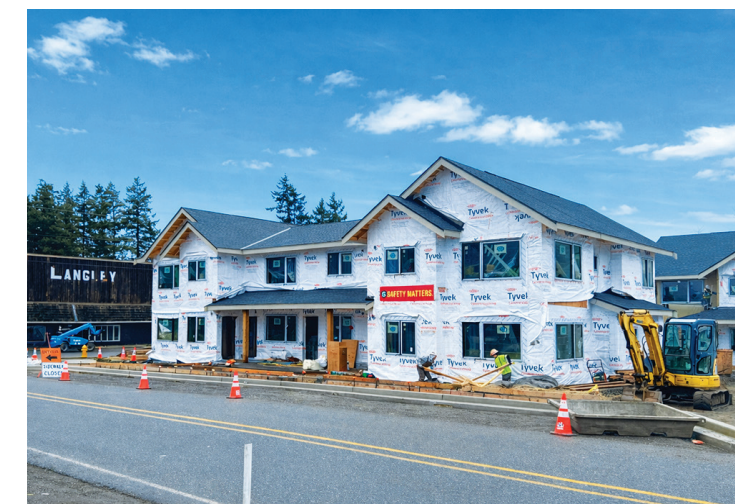
Generations Place construction is underway on 14 family-sized apartment units for workforce rental housing.
